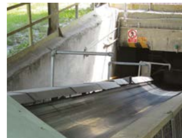
System of sprinklers alongside the RHC115 conveyor
